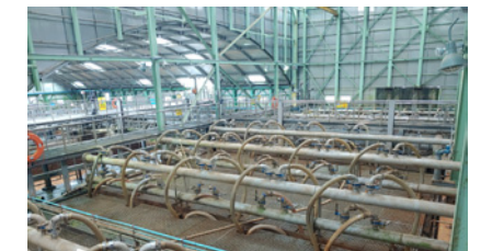
Guri Sewage Treatment Facility Beneficiary: Guri City Capacity: 26,000m 3 /day
