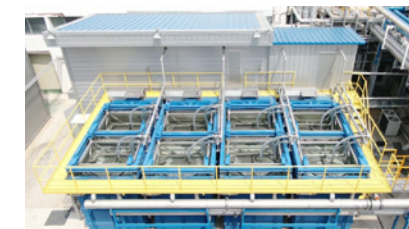
KOLON Glotech Wastewater Treatment Facility Beneficiary: KOLON Glotech Co., Ltd. Capacity: 3,300m 3 /day
