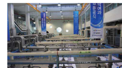
Yeongdeungpo Membrane Filtration Demonstration Water Purification Plant Beneficiary: Seoul Metropolitan City Capacity: 25,000m 3 /day
