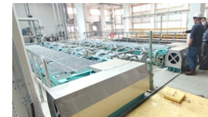
Gumi Group-Wise Wastewater Treatment Facility Beneficiary: KOLON Industries Co., Ltd. Capacity: 10,000m 3 /day
