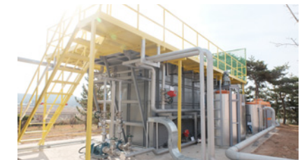
Muan Cheonggye Tertiary Treatment Facility Beneficiary: Muan County Capacity: 1,600m 3 /day
