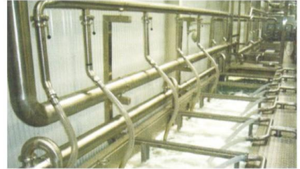
Drinking Water Treatment Plant in Nongfu, China Client ----- Nongfu Spring co., China Capacity ----- 6,720m 3 /day
