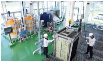
Jeungpyeong Industrial Complex Wastewater Treatment Plant Client ----- Jeungpyeong City Capacity ----- 2,500m 3 /day
