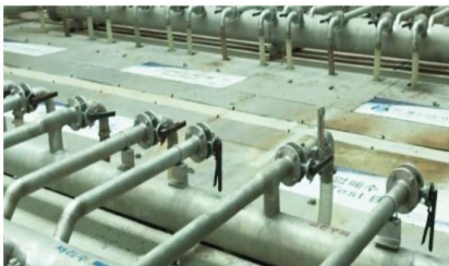
Gumi K Factory Wastewater Treatment Plant Client ----- K company Capacity ----- 10,000m 3 /day
