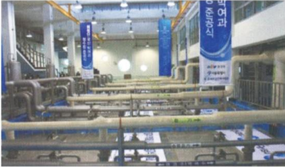
Yeongdeungpo Drinking Water Treatment Plant in Seoul Client ----- Seoul City Capacity ----- 25,000m 3 /day
